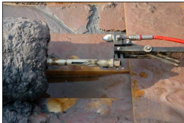
Pulling the long delay fuse with the manipulator
